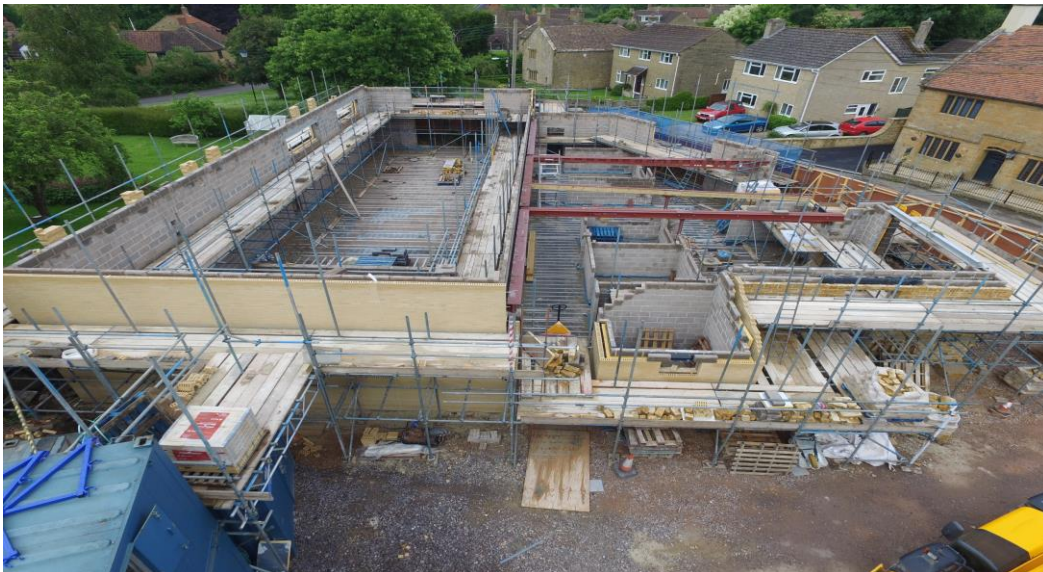
Photo 1. Shows structure up to wall plate level with supporting steelwork in place
